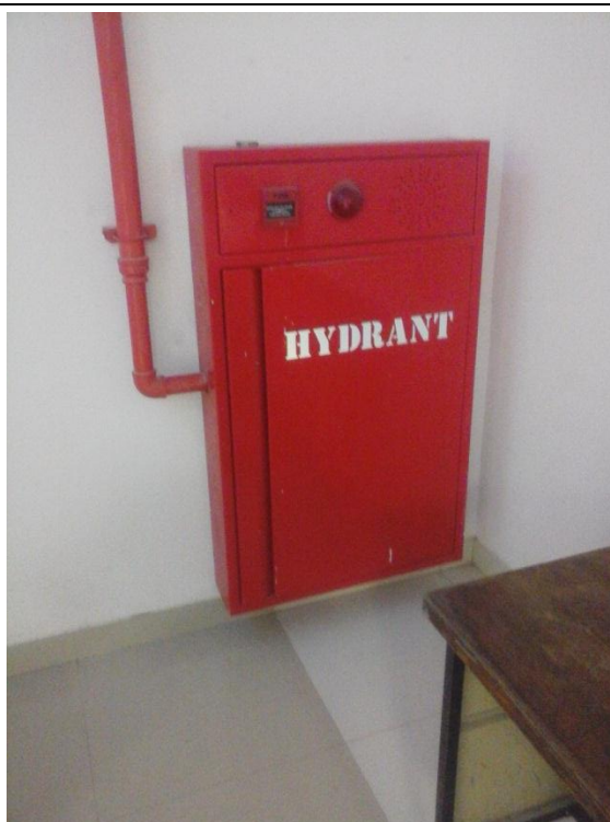
Gambar F.85 Hydrant
