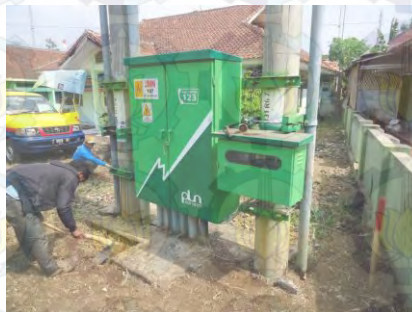
Gambar 2.2 Panel Distribusi PLN
