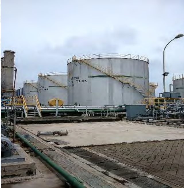
Gambar 2.7. RAW Water Tank
