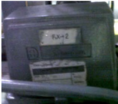
Flow Steam Transmitter FX-2
