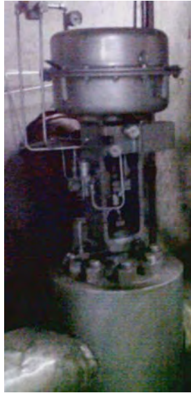
Feed Water Control Valve
