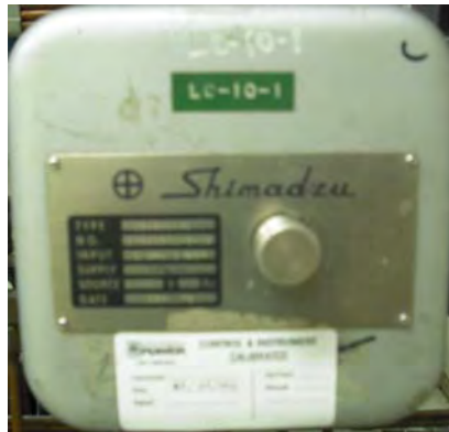
Level Controller LC-10-1
