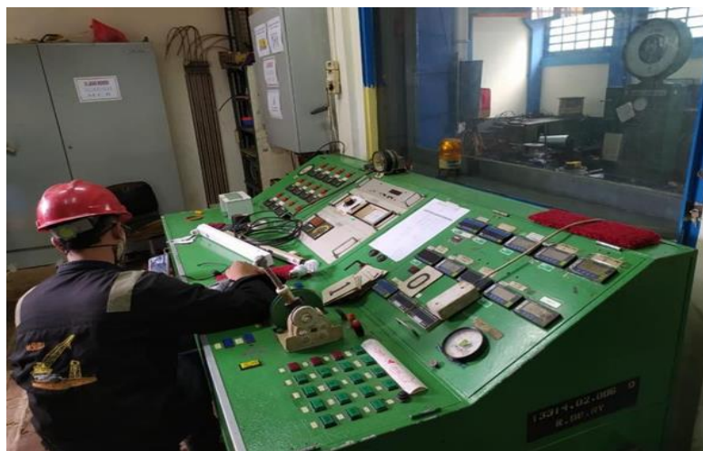
Gambar 2.5 Engine Control Room
