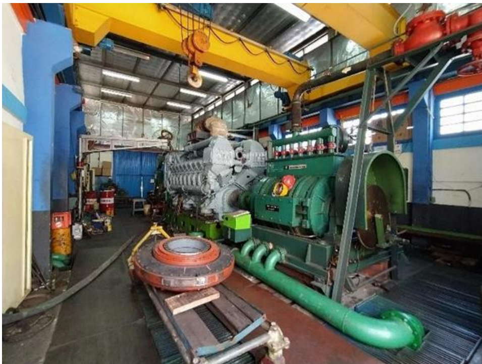
Gambar 2.1 Bengkel Uji Motor (Test Bench)
