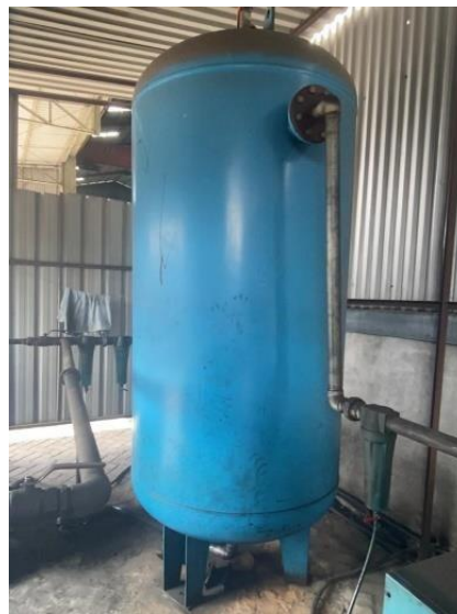
Gambar 4.29 High Pressure Air Receiver Tank
