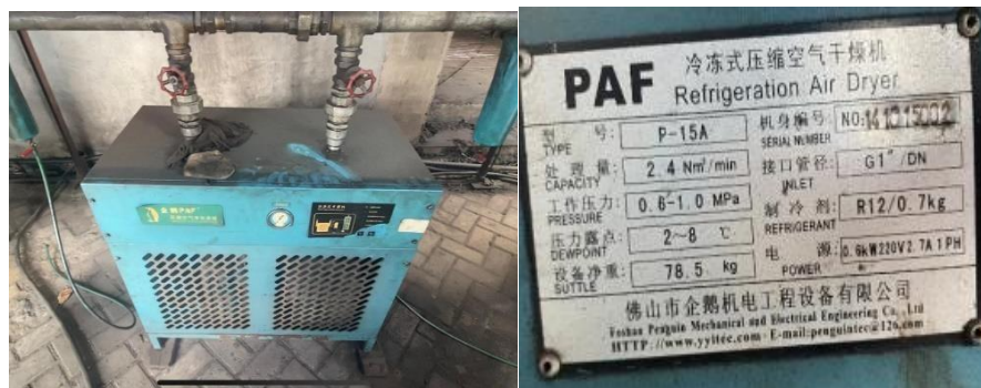
Gambar 4.27 Refrigeration Air Dryer
