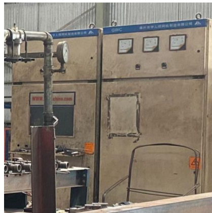
Gambar 4.23 Control System Panel
