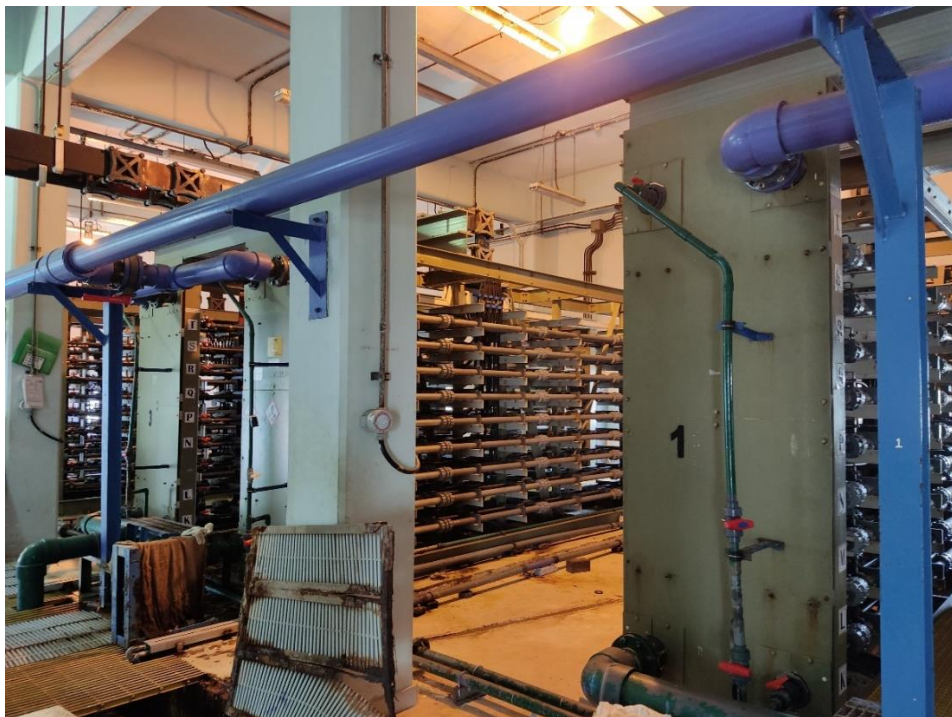
Ruang Chlorination Plant
