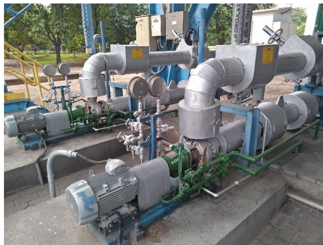
Gambar 4. 25 Low Pressure Boiler Circulating Pump
