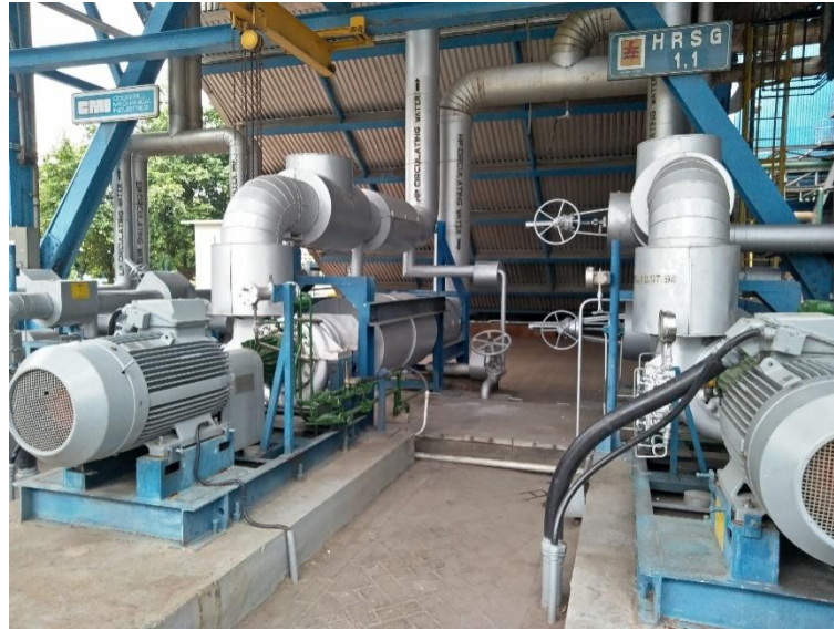
Gambar 4. 12 High Pressure Circulating Pump
