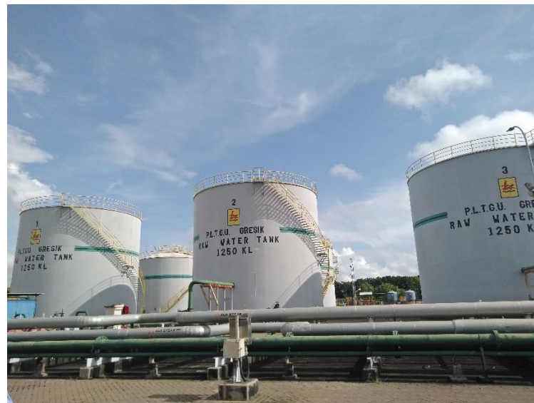
Gambar 4. 15 Raw Water Tank
