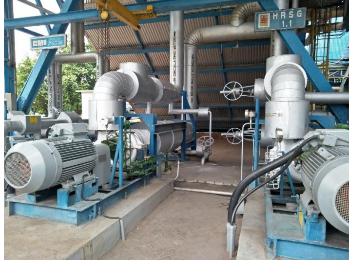
Gambar 4. 27 High Pressure Circulating Pump
