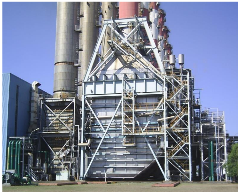
Gambar 4. 7 Heat Recovery Steam Generator
