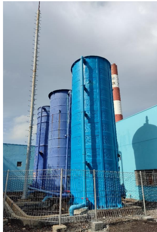
Tangki Chlorination Plant
