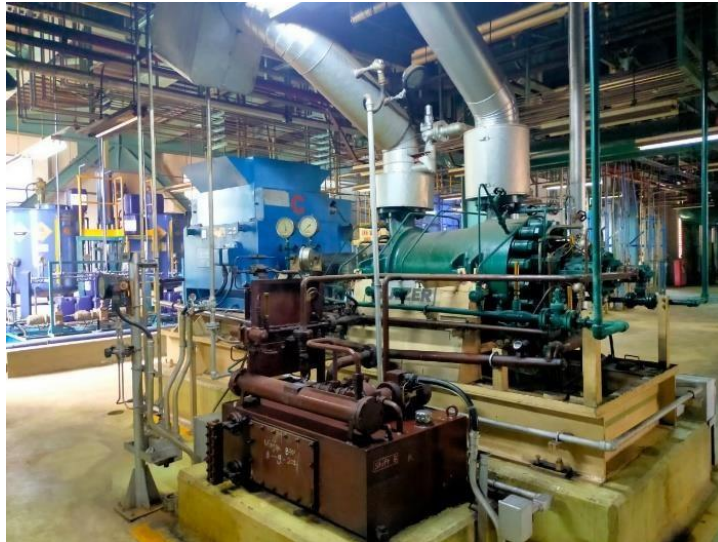
Gambar 4. 10 High Pressure Boiler Feed Pump
