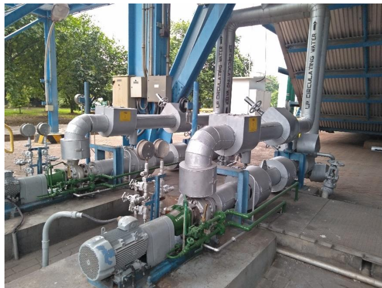
Gambar 4. 11 Low Pressure Circulating Pump
