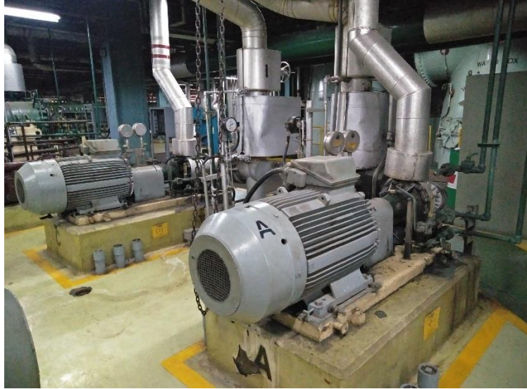
Gambar 4. 9 Low Pressure Boiler Feed Pump
