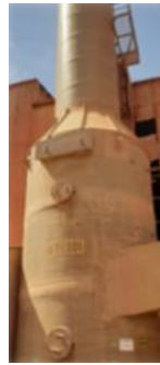
Gambar 4. 12 Tail Gas Scrubber
