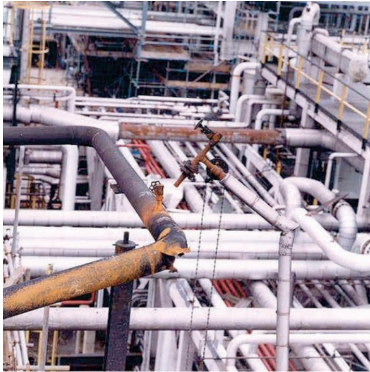
Figure 2. 2 The Failed Pipe Elbow Caused by Corrosion (Source: Jonathan Carter, et al, 200)
