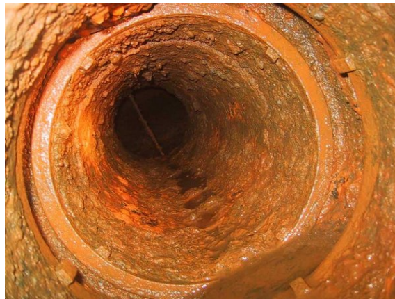
Figure 2. 12 Piping Internal Corrosion (Source: https://pipingengineer.com )
