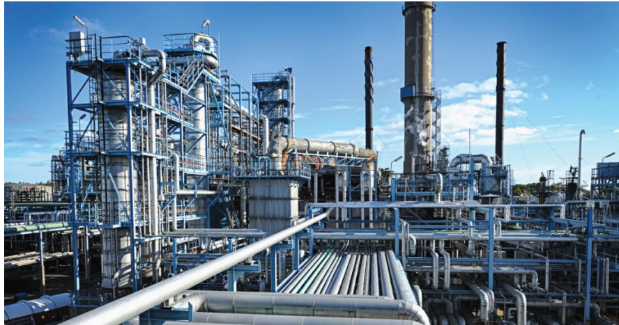
Figure 2. 10 Piping System at CPF (Source: https://www.codesteel.com )
