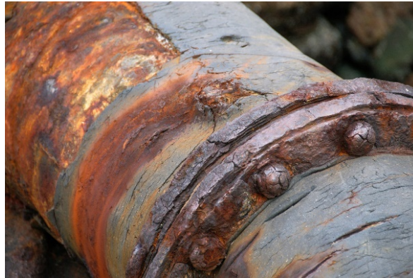
Figure 2. 13 Piping External Corrosion (Source: https://dynagard.com )
