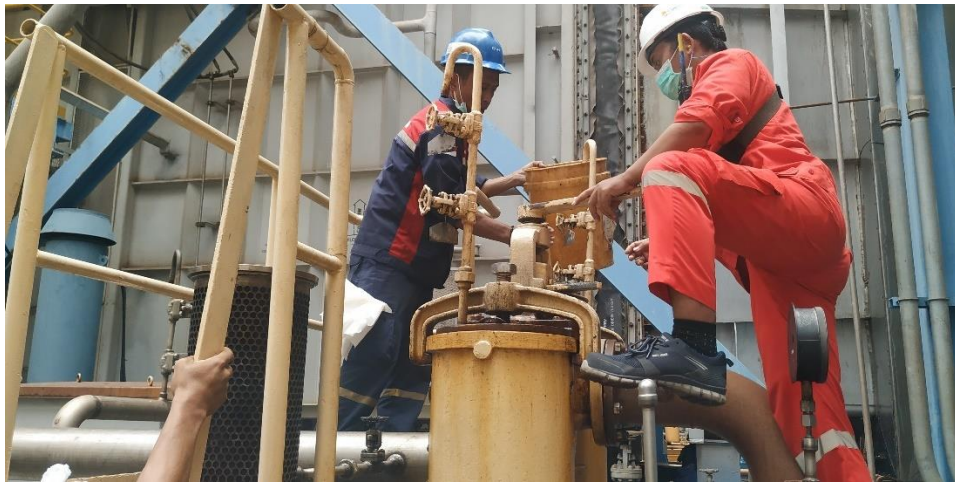
Gambar 4.23 Pelaksanaan Preventive Maintenance Flushing MFOP (main fuel oil pump)
