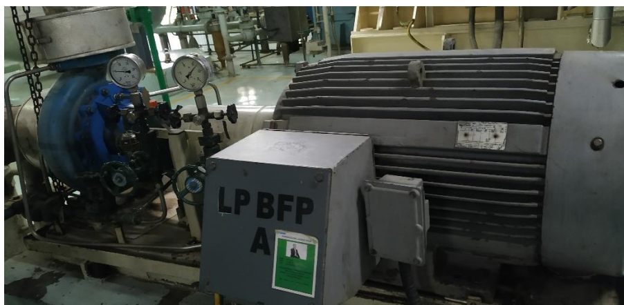
Gambar 4.17 Pompa LP BFP (Low Pressure Boiled feed Pump)
