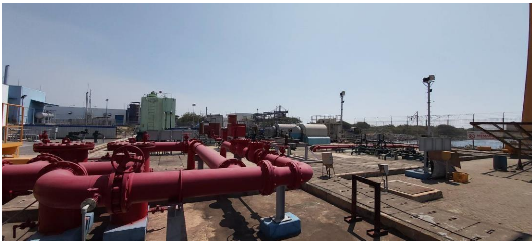
Gambar 4.21 Sea Water Intake
