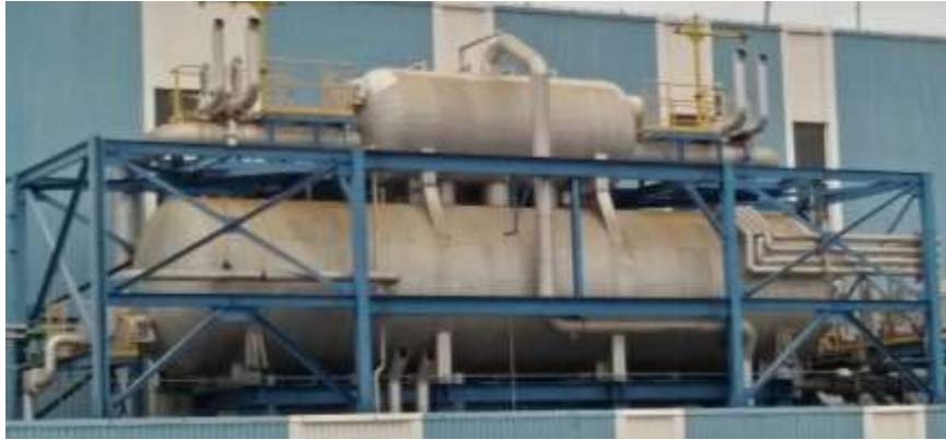
Gambar 4. 9 Deaerator (Sumber : PT. PJB )
