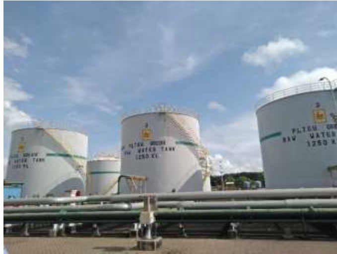
Gambar 4. 6 Raw Water Tank
