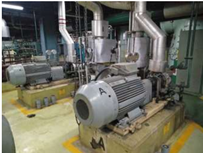
Gambar 4. 13 Low Pressure Boiler Feed Pump PLTGU UP Gresik (Sumber : PT. PJB )
