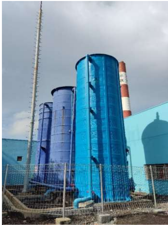
Tangki Clorination Plant
