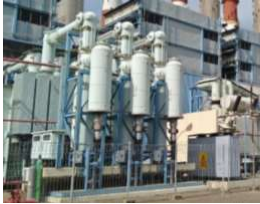
Gambar 4. 10 Transformator (Sumber : PT. PJB )
