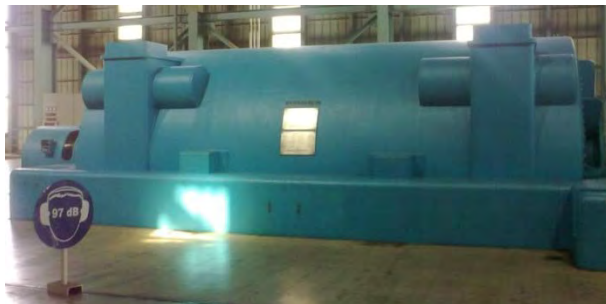
Gambar 2.4 Generator PLTU unit 4
