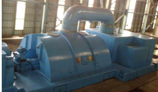
Gambar 2.2 Turbin PLTU Unit 4
