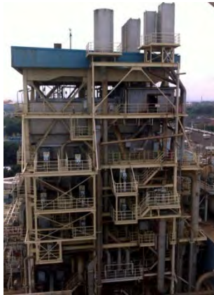
Gambar 2.1 Boiler PLTU Unit 4
