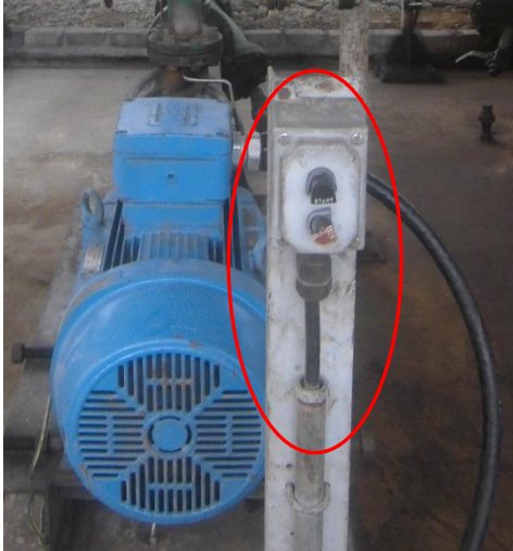
Gambar 4.14 Instalasi kelistrikan crude oil booster pump
