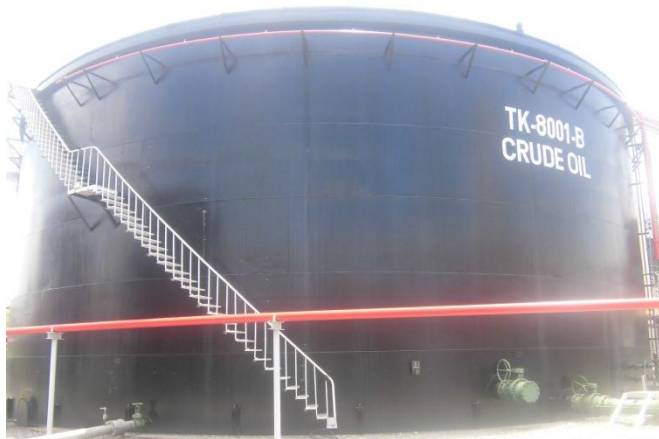
Gambar 4.13 Crude oil tank (TK-8001B)
