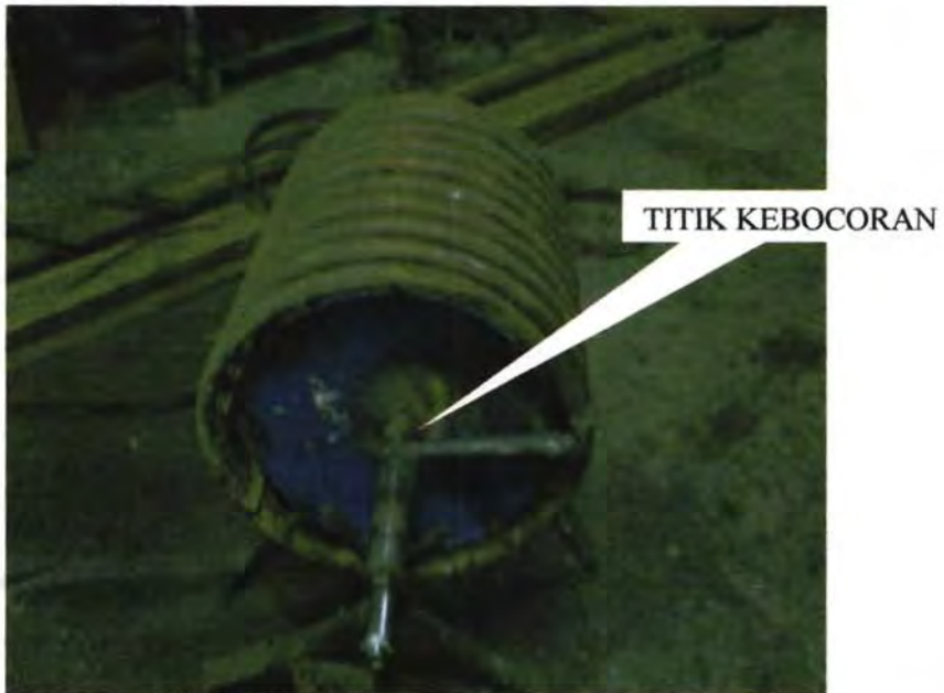
Gambar 5.3 kebocoran pipa evaporator
