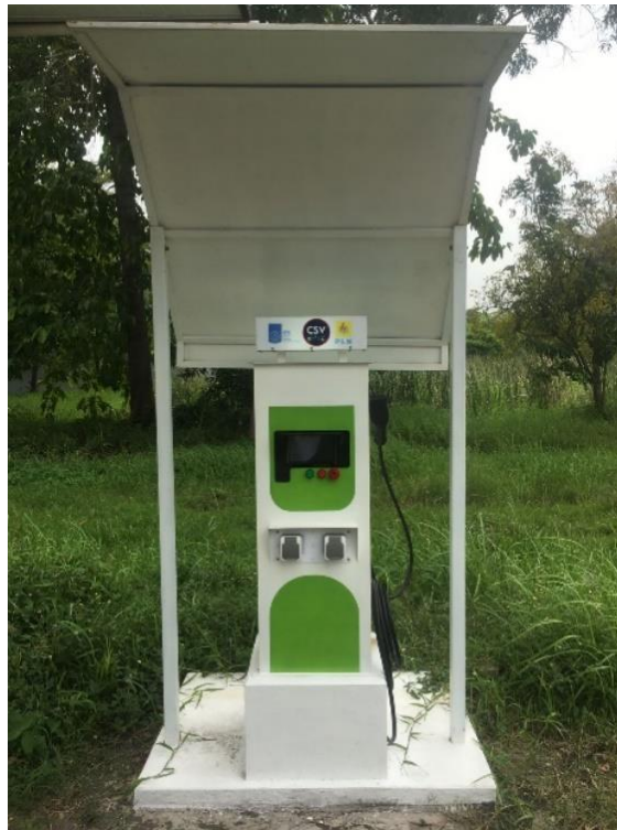
Gambar 2. 12 Smart Charging Station
