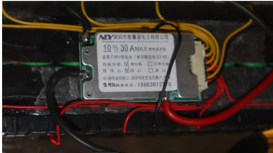
Gambar 4.9 BMS ( Battery Management System )
