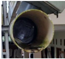
Figure 4. 2 The Rain Gutters of the Male Dorm in Condition
