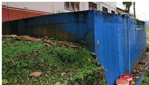
Figure 2. 4 Communal Reservoir in Al Kahfi Islamic Boarding School
