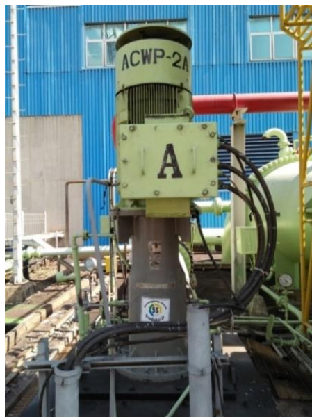
Gambar 5.44 Auxiliary Cooling Water Pump
