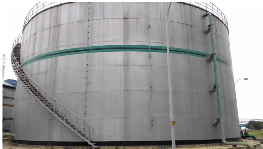
Gambar 5.55 Well Water Tank
