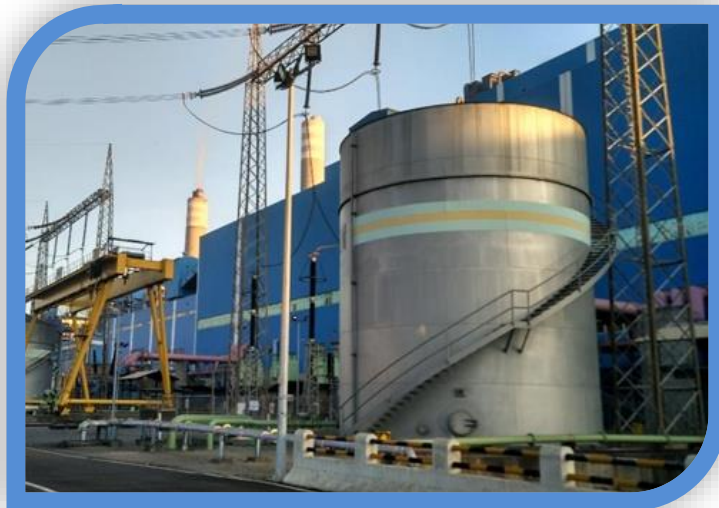
Gambar 5.48 Condesansate Storage Tank
