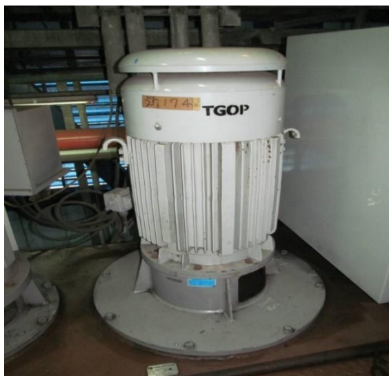
Gambar 5.51 Turning Gear Oil Pump
