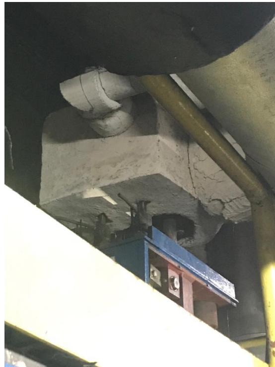
Gambar 5.21 Seal Steam Header
