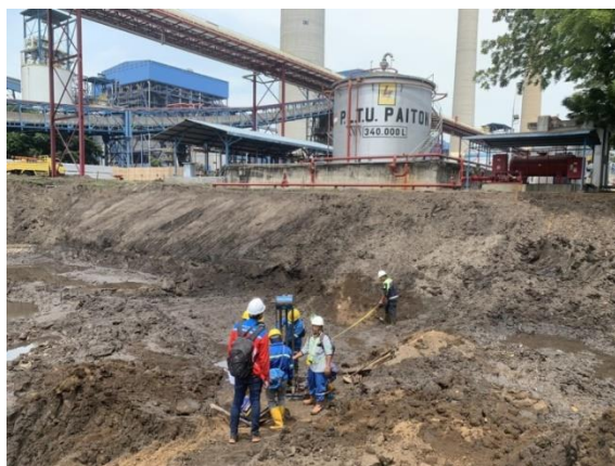
Gambar 5.63 Metal Cleaning Waste Water Treatment Plant
