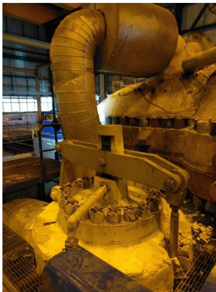
Gambar 5.25 Reheat Valve dan Interceptor Valve
