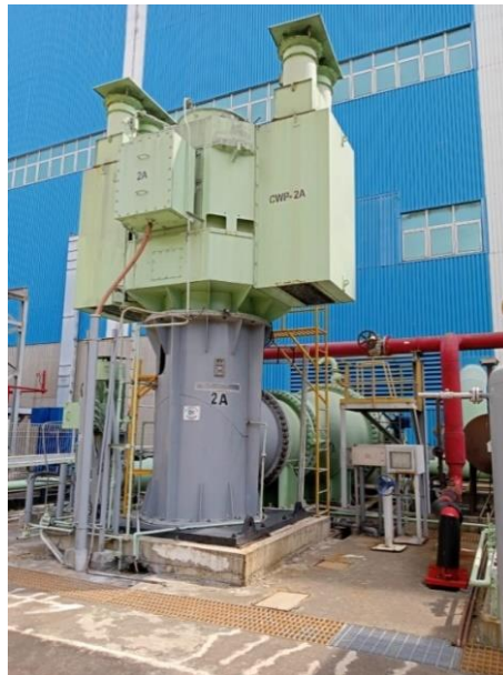
Gambar 5.43 Cooling Water Pump
