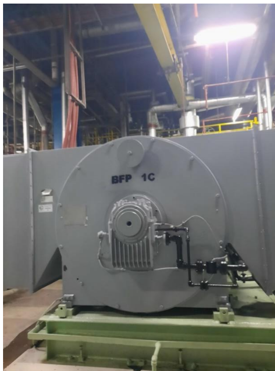
Gambar 5.6 Boiler Feed Pump
