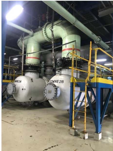
Gambar 5.45 Closed Cooling Water Heat Exchanger
