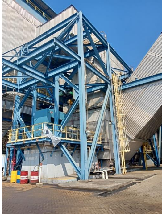
Gambar 5.33 Induced Draft Fan
