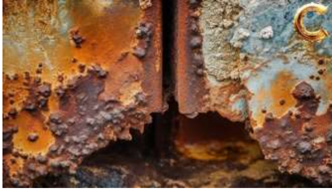
Gambar 2.11 Contoh pitting corrosion (Ali, 2016)
