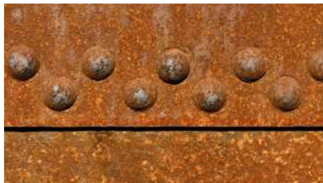
Gambar 2.10 Contoh Surface Corrosion (Rosyidin, 2016)
