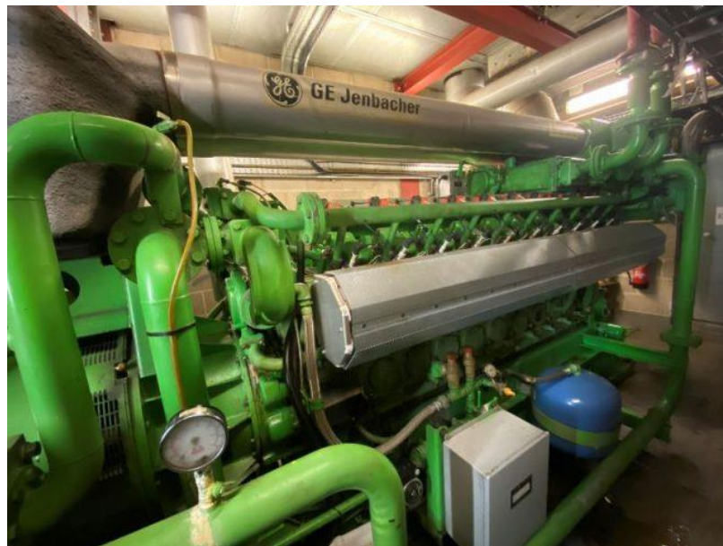
Gambar 2. 27 Gas Engine (Sumber : www.generalelectric.com )
