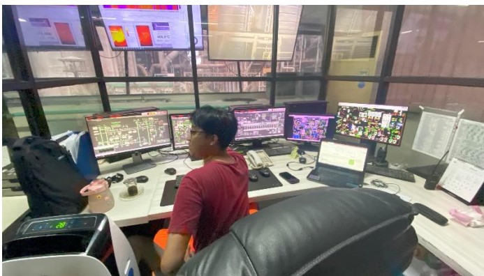
Kiln Operation Control Room
