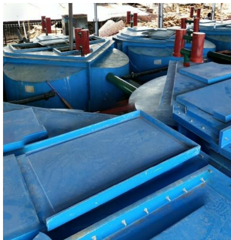
Gambar 2. 5 Unit Biofilter Anaerobik
