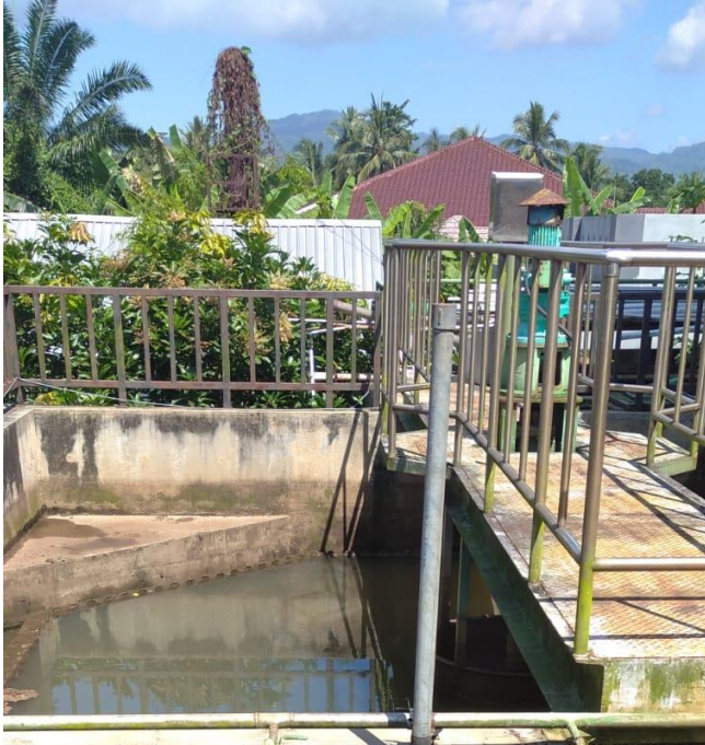
Unit Sedimentasi II IPAL RSUD Banyumas
