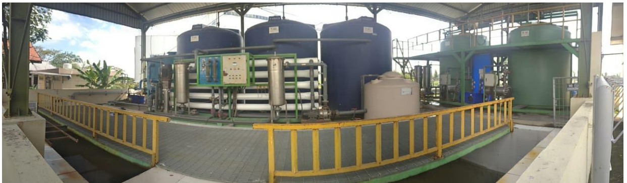
Instalasi Pengolahan Lindi TPA Benowo
