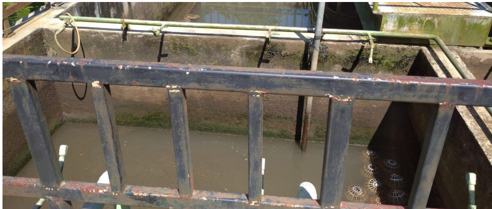
Unit fluidized bed biofilter reactor IPAL RSUD
