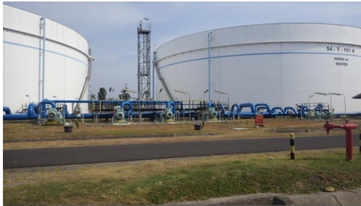
Gambar 4. 5 Service Water Tank (Sumber ; Pertamina, 2009)
