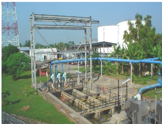
Gambar 4. 4 Water Treatment Plant Salamdarma (Sumber : Modul WTP Salamdarma)
