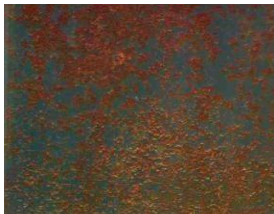
Gambar 2.18 Rust Grade B (ISO 8501, 2011)
