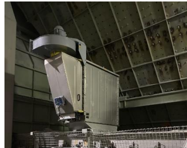
Gambar 4. 32 Dust Collector Unit
