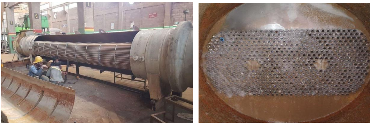
Gambar 10 Kerusakan Heat Exchanger Shell & Tube
