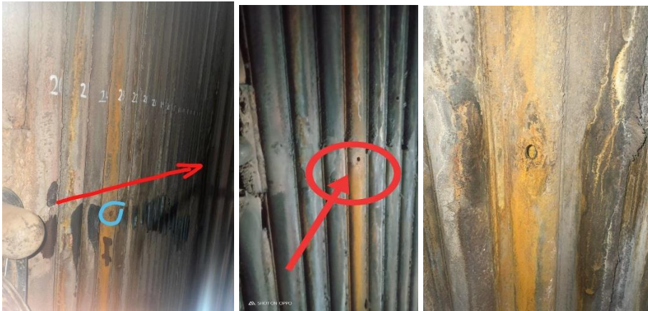
Gambar 4.2 Visual inspeksi kegagalan rear water wall tube elevasi 29.8 mdpl (area Sootblower IR20)
