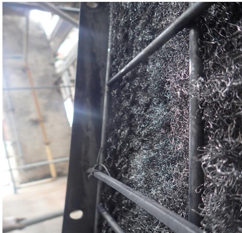
Gambar 4.11 Ketebalan Wire demister berkurang
