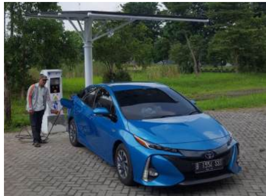
Gambar 2.31 PV Charging Station
