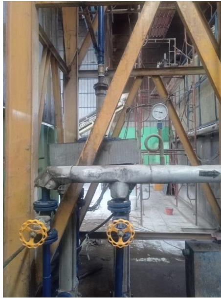
Gambar 4. 3 Pompa Umpan ( Feed Water Pump ) (Sumber: Dokumentasi Pribadi)
