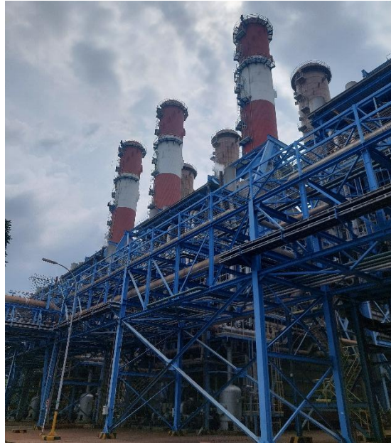
Gambar 4. 17 Heat Recovery Steam Generator Blok 2.3
