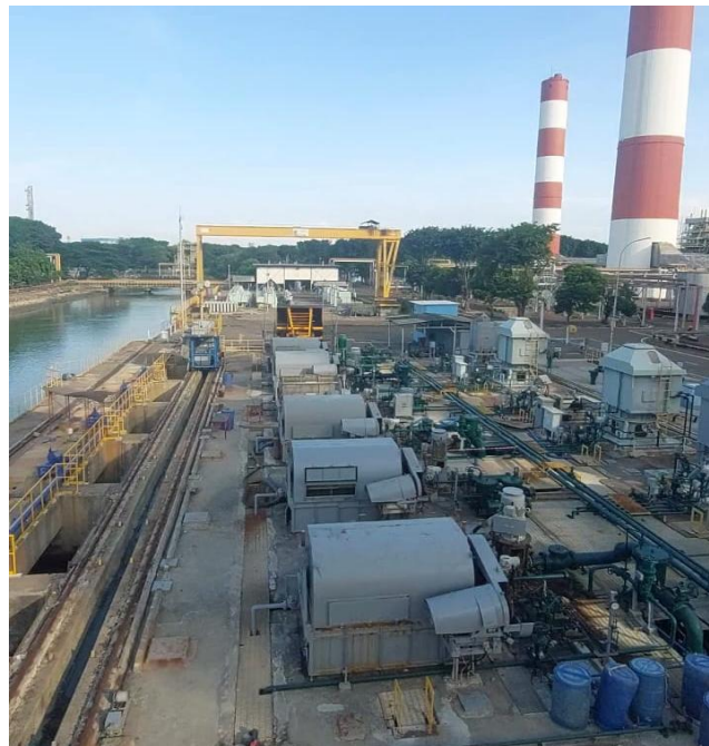
Gambar 4. 23 Sea Water Intake
