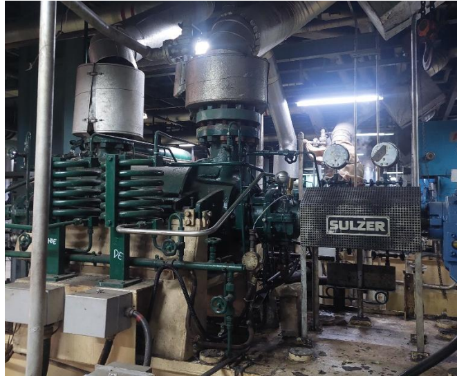
Gambar 4. 15 Pompa HP BFP ( Hight Pressure Boiler Feed Pump )
