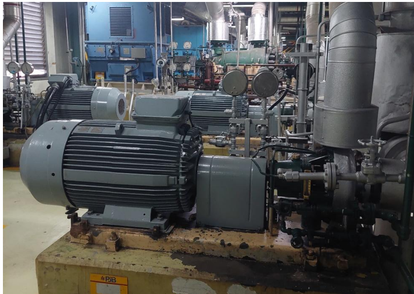
Gambar 4. 16 Pompa LP BFP ( Low Pressure Boiler Feed Pump )
