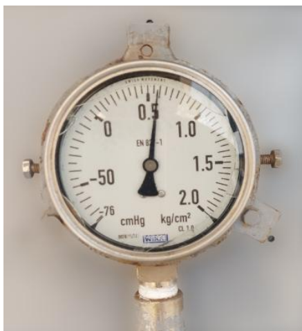
Gambar 4. 41 Discharge Pressure Pompa CWP Sebelum Overhaul
