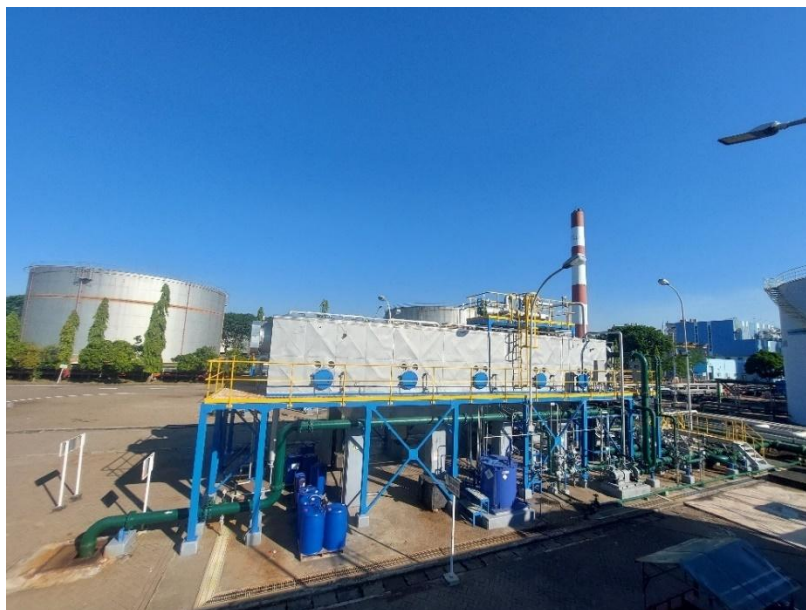
Gambar 4. 18 Desalination Plant Area
