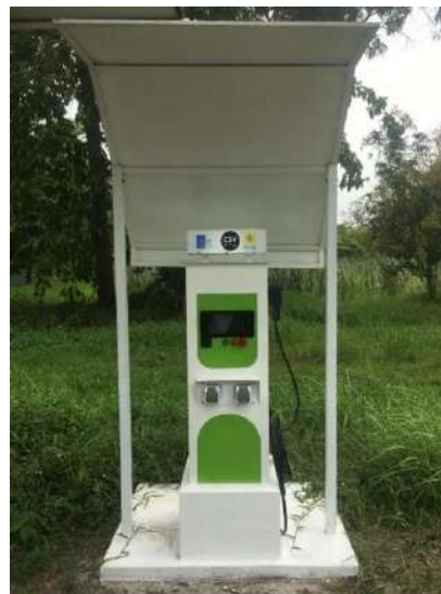
Gambar 2. 17 Smart Charging Station
