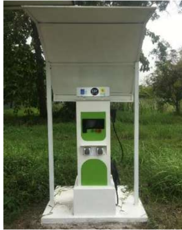
Gambar 2.33 Smart Charging Station
