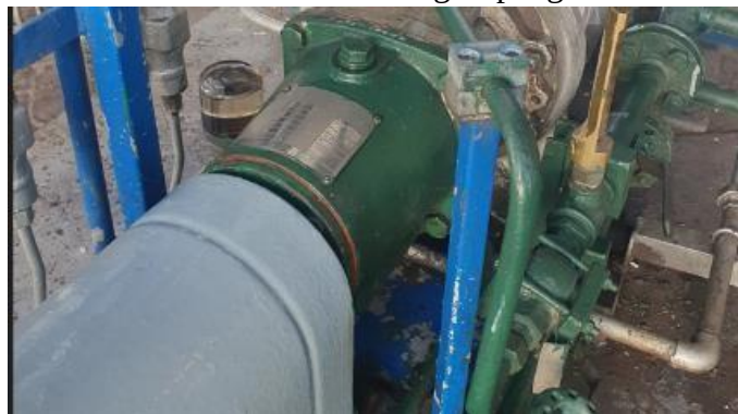
Gambar 4. 39 HP(High Pressure)-LP(Low Pressure) BCP(Boiler Circulating Pump)
