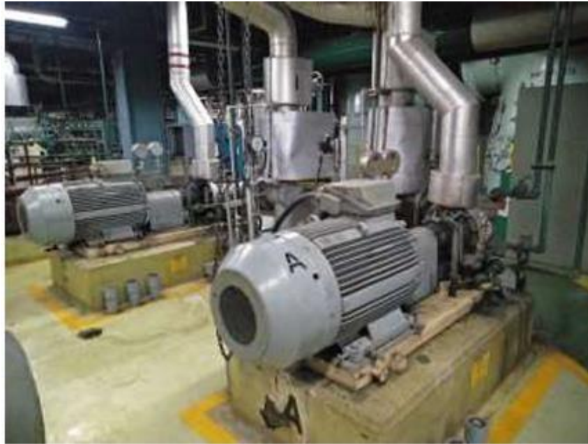
Gambar 4. 10 Pompa LP BFP (Low Pressure Boiler Feed Pump)
