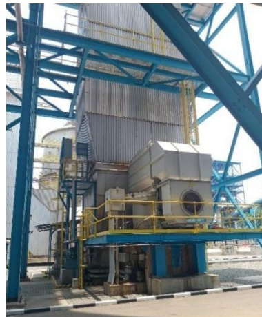
Gambar 4. 9 Induced Draft Fan
