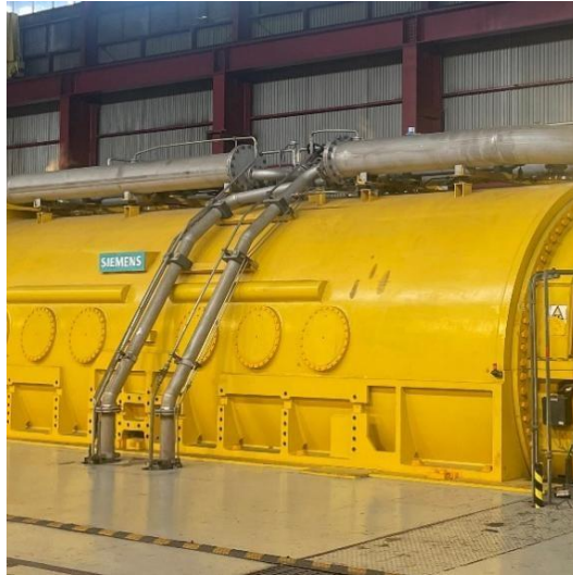
Gambar 4. 15 Low Pressure Turbin
