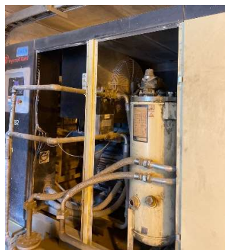
Gambar 4.20 Observasi Unit Compressor
