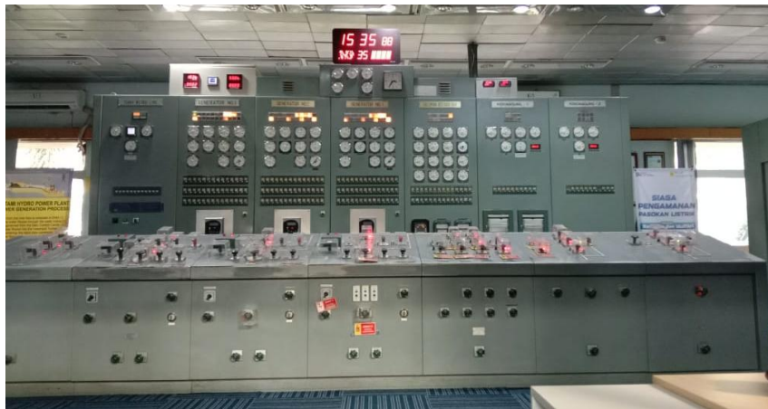
Gambar 4.20 Ruang Center Control Room (CCR)
