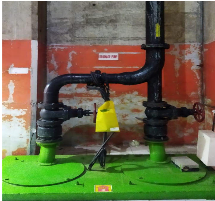
Gambar 4.16 Sistem Pengurasan ( Drainage System )
