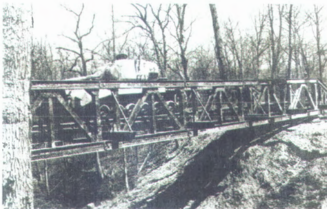
Figure 2-8. T8 aluminum flood bridge.
