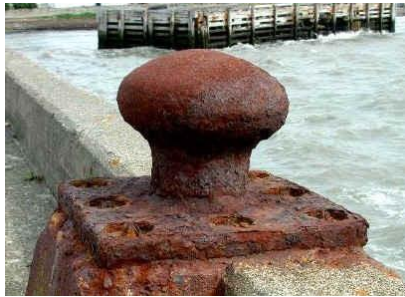
Gambar 2.3 Korosi Uniform (API 571)
