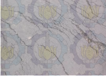
Gambar 2. 7 Retak selip (Slippage cracks)
