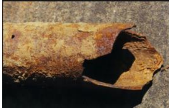
Gambar 2. 2 Korosi Merata ( Corrosionclinic, 2013 )
