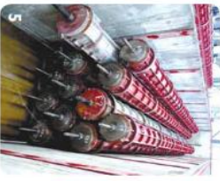
STEAM CURING The pile is then subjected to steam curing process in order to achieve the required transfer strength for early demoulding.
