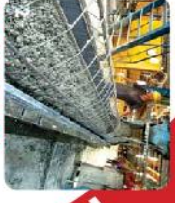
CONCRETE FEEDING Concrete from the compressed batching plant is discharged into a feeding hopper. Concrete is then fed into the bottom half mould. The top half mould is then tilted to the bottom half.
