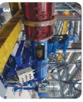
STRESSING The bars are tensioned around the mould through the ends and stressing plate. The stressing is being carried out in a single operation. This ensures uniformity of stress in all the PC bars and hence straightness of the pile.
