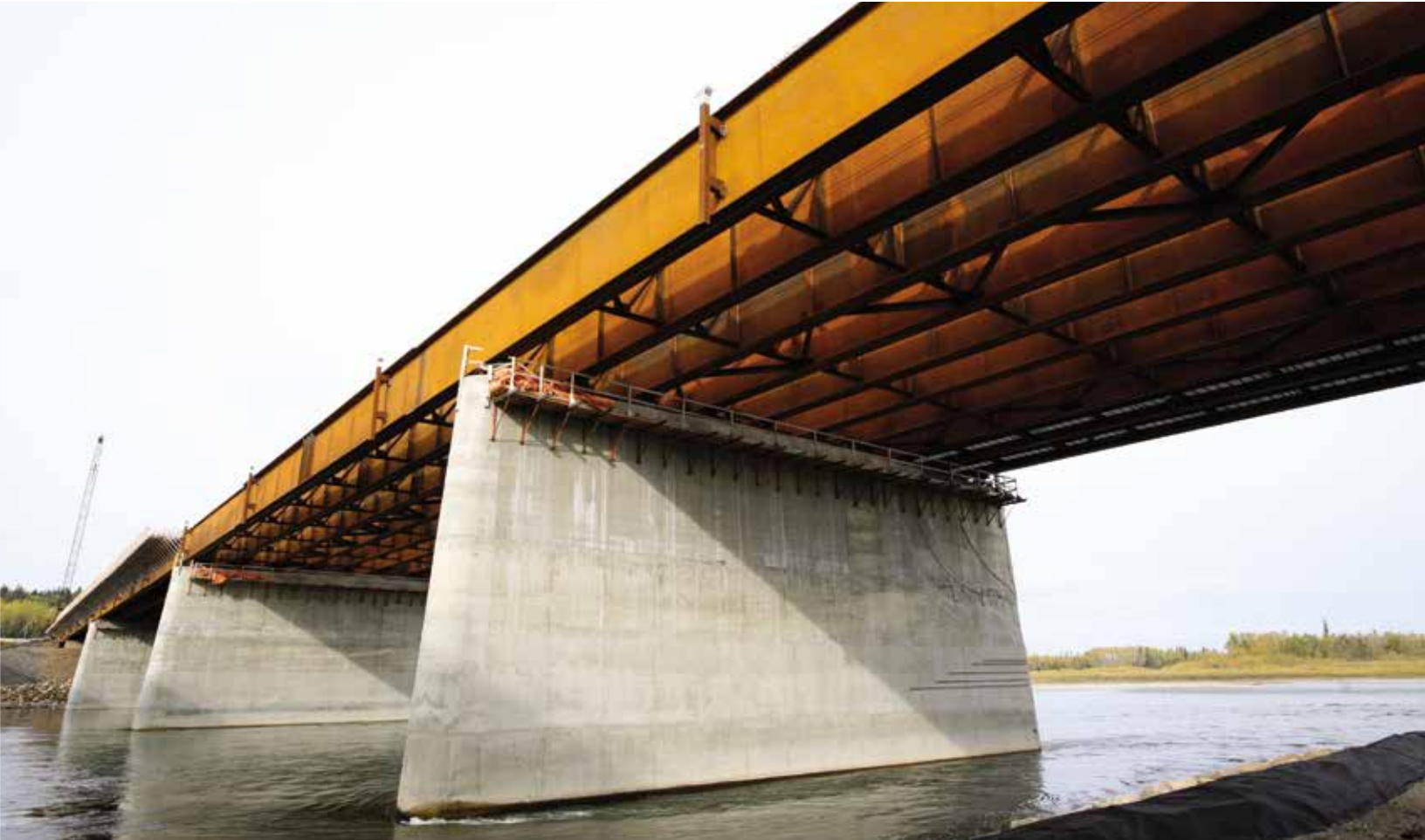
Athabasca River Bridge – Fort McMurray, AB With a deck surface of 15,500 m 2 (166,841 sq. ft.), this is Alberta’s widest bridge.
