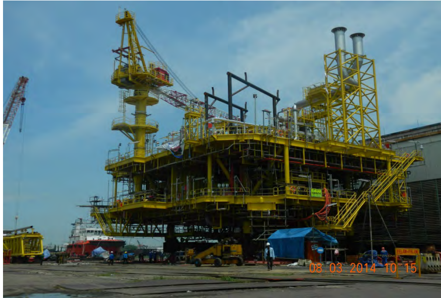
Gambar II.2 Banuwati Topside Deck (Sumber : PT.PAL Indonesia)
