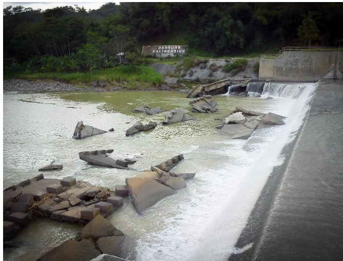
Gambar 1.2 Kerusakan Kolam Olak di Bendung Kaligending ( https://myfreakysunday.wordpress.com/2014/11/02/river-explorer/ )
