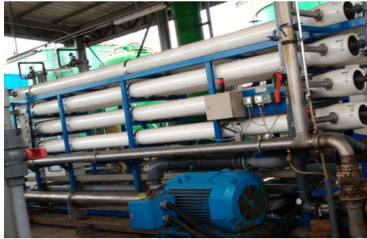
Gambar 2.4 Desalination System Tipe Reverse-Osmosis PLTU Belitung
