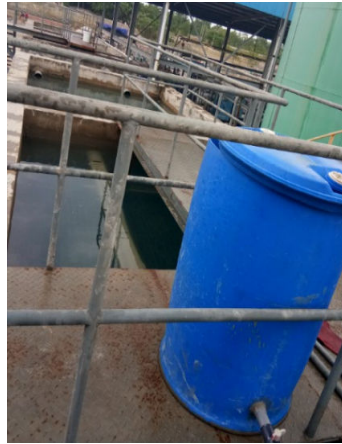
Gambar 2.8 Injeksi Koagulan-aid di Inlet Clarifier PLTU Belitung
