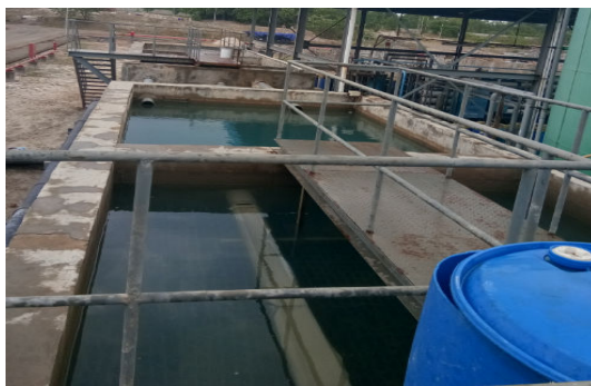
Gambar 2.3 Pre-Treatment Water System Tipe Lamella Clarifier PLTU Belitung
