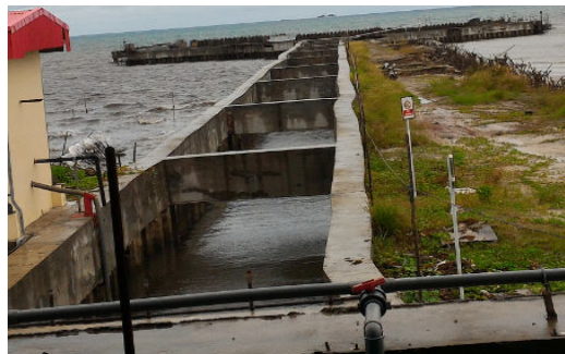
Gambar 2.2 Sea Water Intake PLTU Belitung
