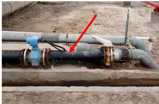
Gambar 2.7 Static Mixer Pipe di Inlet Clarifier PLTU Belitung
