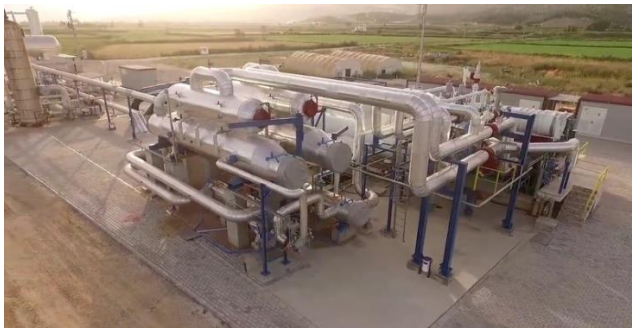
Gambar 1.2. Akça Binary Geothermal Power Plant kapasitas 4 MW
