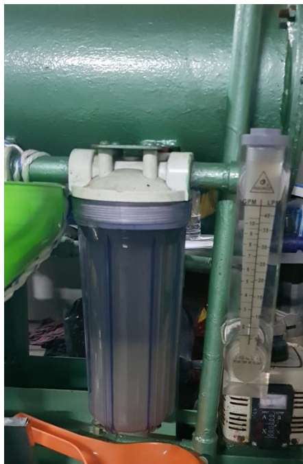
Figure 26 Crumb rubber was pushed upwards resulting to flow drops.
