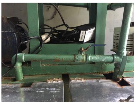
Figure 15 The new pipeline from output line, bypassed to the input tank.
