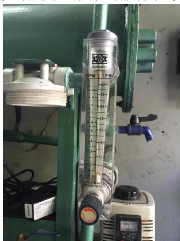
Figure 14 New flow meter installed on the prototype.
