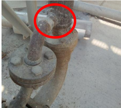
Gambar 4.6 Line steam jacket bocor
