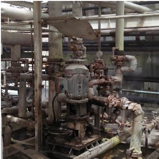
Gambar 2.16 Pompa P-1002 A/B Unit Sulphur Handling
