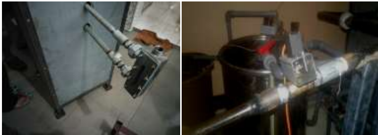
Gambar 4.2 A: Level Sight Glass. B: Servo Operating Valve
